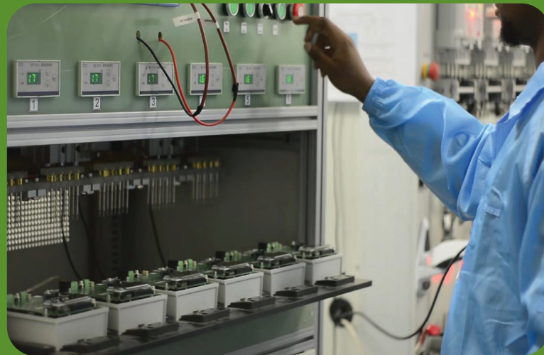
High Voltage testing
